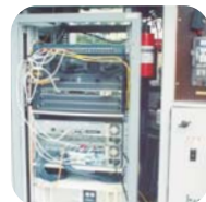
Telecommunication Equipment Cabinet
